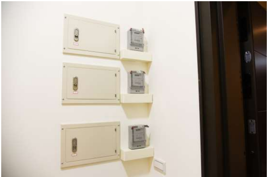
房間電表 Electricity Meter in the Room
